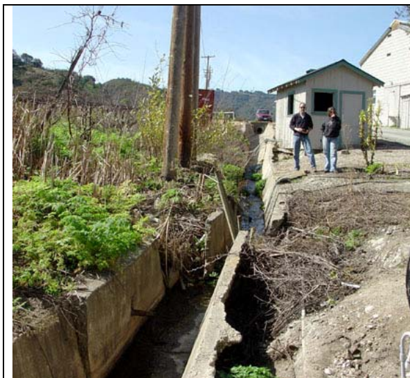
Figure 2-7. This cement-lined drainage ditch on the south side of the DeRose Vineyards shows offset from creep along the San Andreas Fault. The drain was probably constructed before the 1906 earthquake.
