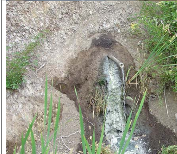
Figure 2-18. A drain pipe in the Santa Cruz Mudstone near the fault zone is a source of sulfur-rich water. Sulfur and mineral springs are common along faults throughout the region. Warning! Do not attempt to have field trip participants cross the road to examine the springs or outcrops. There isn't enough room to stand next to the road. Rather, a single individual might carefully cross the road and fill a water jug. However, the rotten-egg smelling water is not safe to drink. Cattails grow in abundance near the springs.
