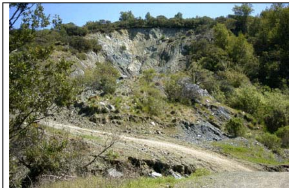
Figure 3-3. An active landslide along the Limekiln Trail causes trail closure during wet seasons. In recent winters the road has been offset by several meters. During dry months the slide area is relatively safe to examine but be aware that rocks and soil in steep slopes may be unstable from recent movement. The landslide formed in deeply weathered serpentinite, but fresh blocks of rock material have accumulated in the stream at the toe of the slump.
